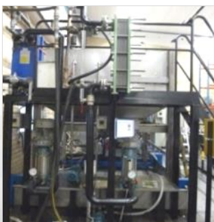
Installed at Wire drawing plant, Sandvik AB
